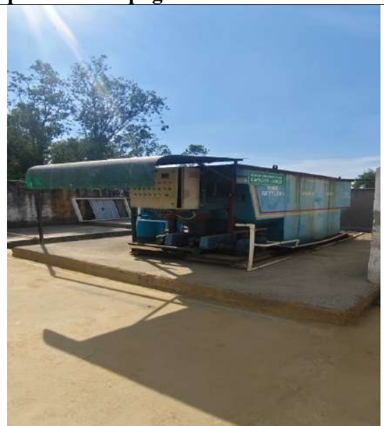
Photograph of STP installed in unit
